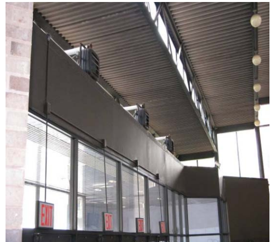
Large amounts of single-pane glass and infiltration in the entry result in a need for the unit heaters shown above.
