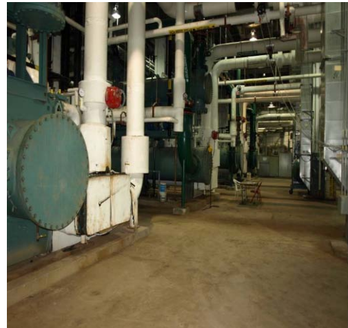
The newly renovated chiller plant.
