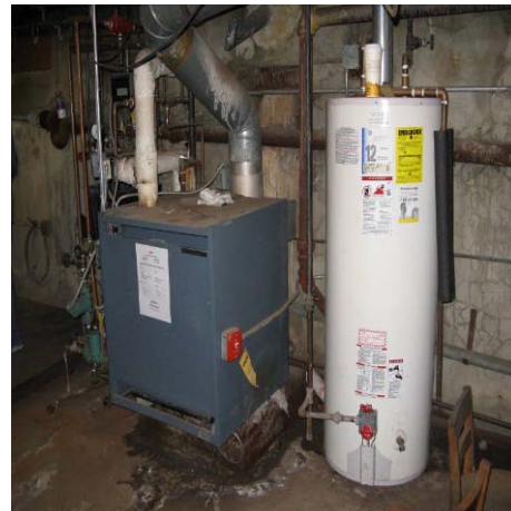
Boiler and water heater
